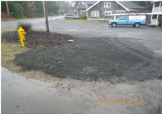
After we replaced the service line & the angle meter stop for the Pilot House.
