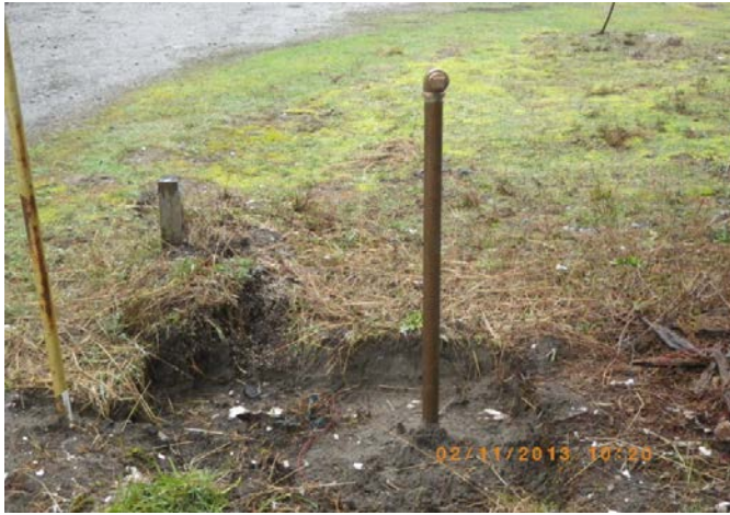
New blow off we installed at the South end of K PI off 225th.
